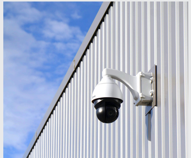
Installed outside an airport terminal, the FLIR Quasar 1080p IR PTZ camera observes, detects and classifies objects up to 200 meters across wide areas in diverse lighting conditions.
