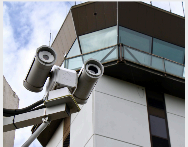
FLIR cameras mounted near SJC’s northern-most control tower expand surveillance coverage.
