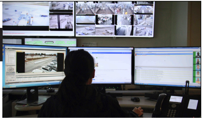
The FLIR Command Center, powered by FLIR Latitude Video Management System, enables easy viewing and simplified management of all FLIR cameras deployed along the perimeter.
